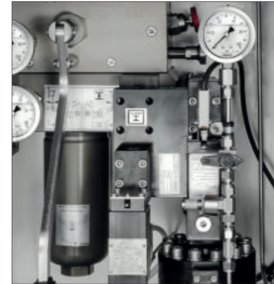
Left: Type KY control with remote control OPEN/CLOSE, incl. - Torque limitation - Automatic pipe fracture response with manual reset and optional adjustment set
